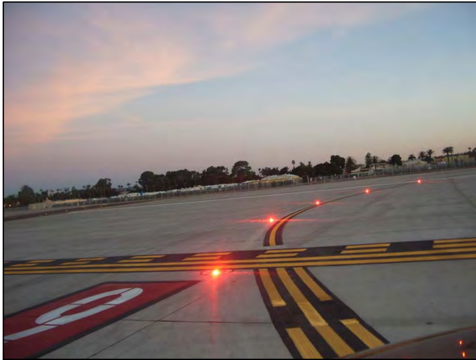
FIG 2-1-12 Runway Entrance Lights
